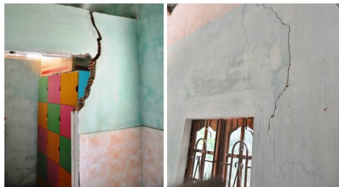
Figure 6. Cracks found on the walls of houses at Song Tranh, Tra My, Vietnam after the earthquake of 5.1 Richter in May 2013
